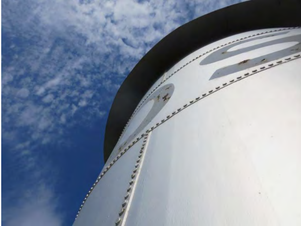
Photo 10 - Tank wall - note pealed paint and rust in letters
