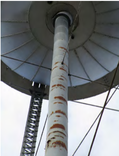
Photograph of riser shaft showing the corroded steel and the insufficient joint between the shaft and the tank.
