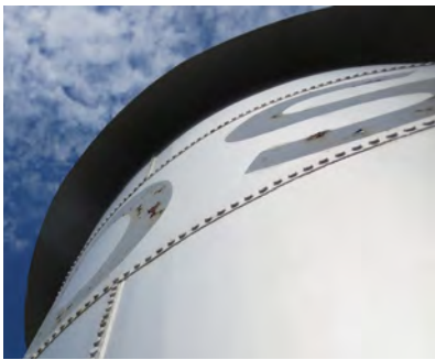
Paint damage on the tank exterior.
