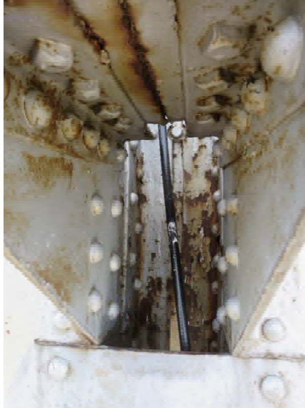
Photo 12 - Support bracket below walkway - surface rust and some deterioration evident
