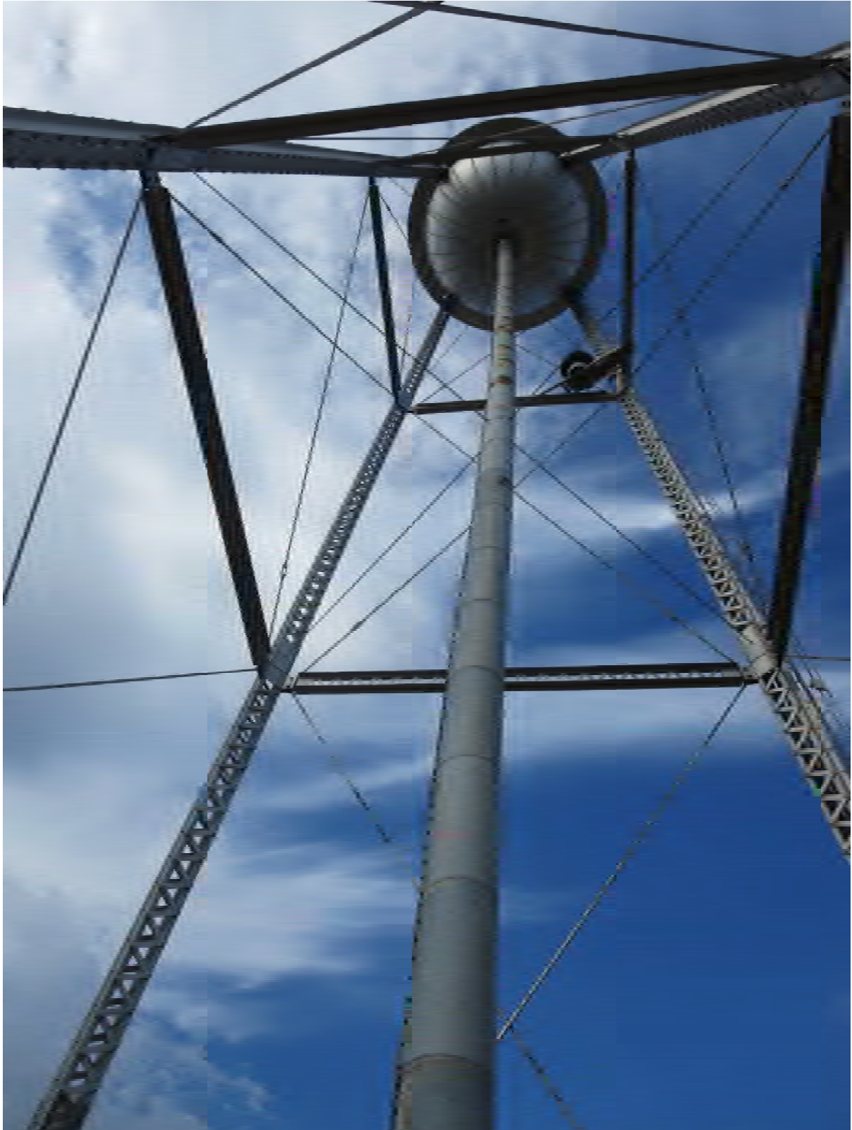
Photo 15 - Base of tank and bracing - note dark spots on bracing are surface rust locations
