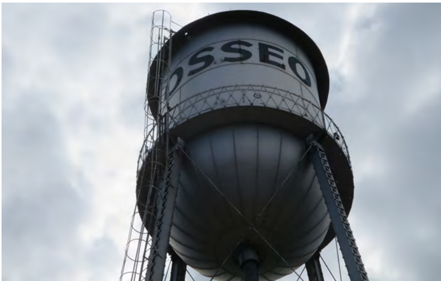
Photograph of the north side of the tower, showing the painted letters and ladder cage.
