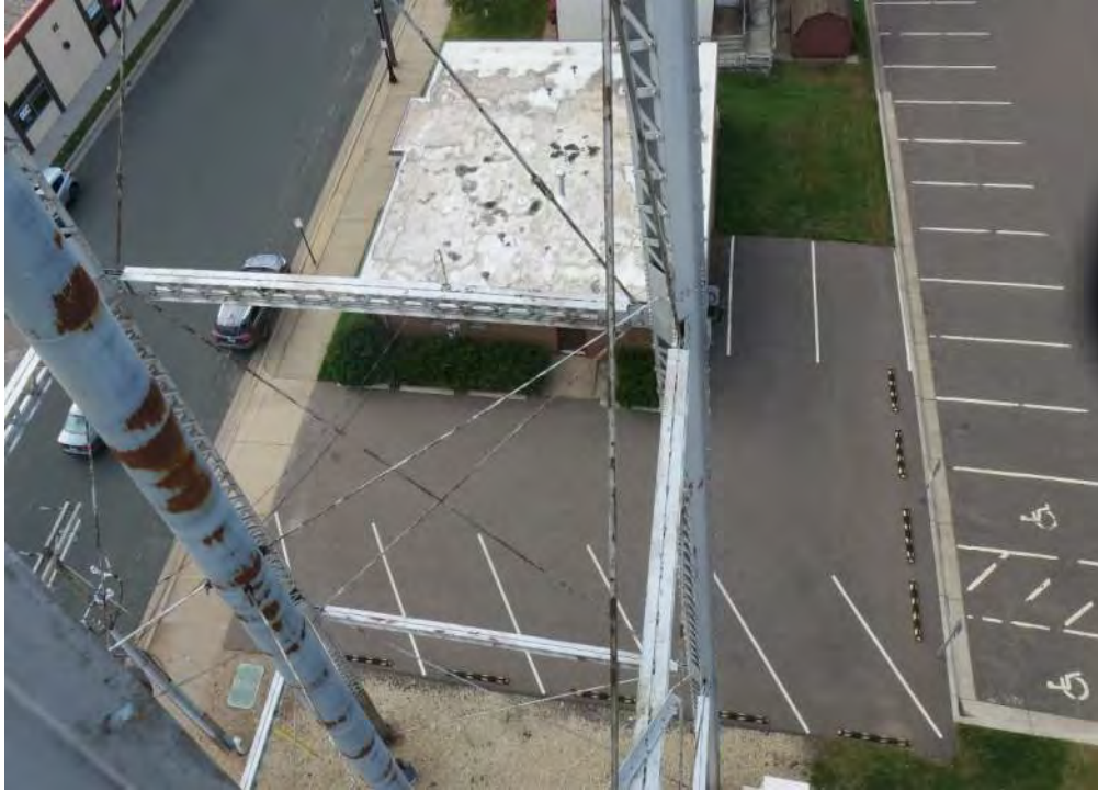
Photo 8 - Looking down at bracing - note rust and deteriorated paint
