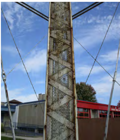
Corrosion at mesh on southwest leg of tower.
