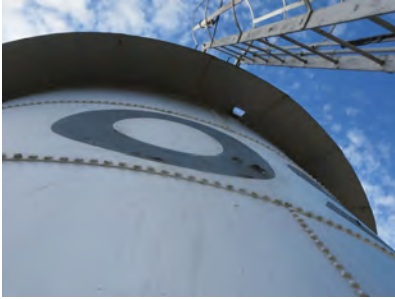
Flaking paint on the “O” on the north side of the tower.
