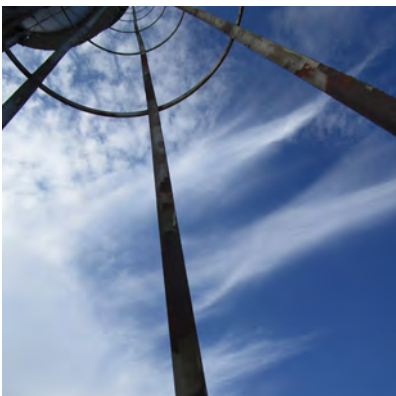
Peeling paint and exposed steel on the ladder cage.
