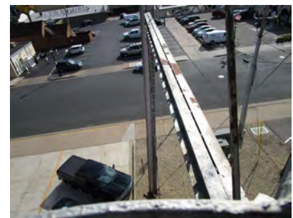
Peeling paint on structure, photograph facing south.
