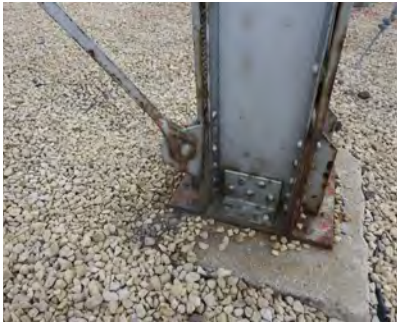
Erosion at southeast concrete footing and corrosion at steel.
