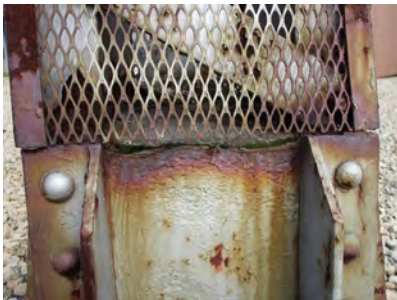
Corrosion and vegetation growth at base of southwest tower leg.
