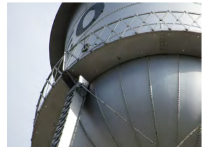
Photograph showing balcony walkway cut out at leg and the guardrail.
