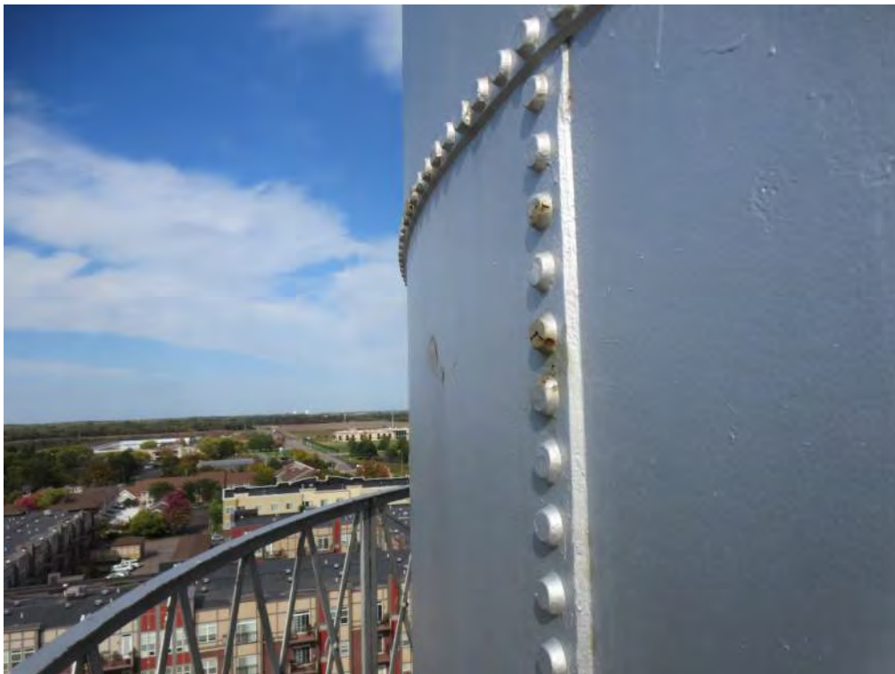
Photo 11 - Tank plate joint - rust evident at some rivets
