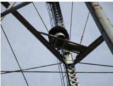
Photograph looking up at the emergency siren and its platform from the ground.
