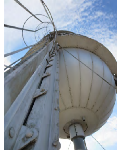
View of the cage ladder on the northeast leg of the tower and the hemispherical tank bottom.
