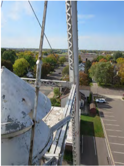
Close up view of emergency siren at northeast corner of the water tower.
