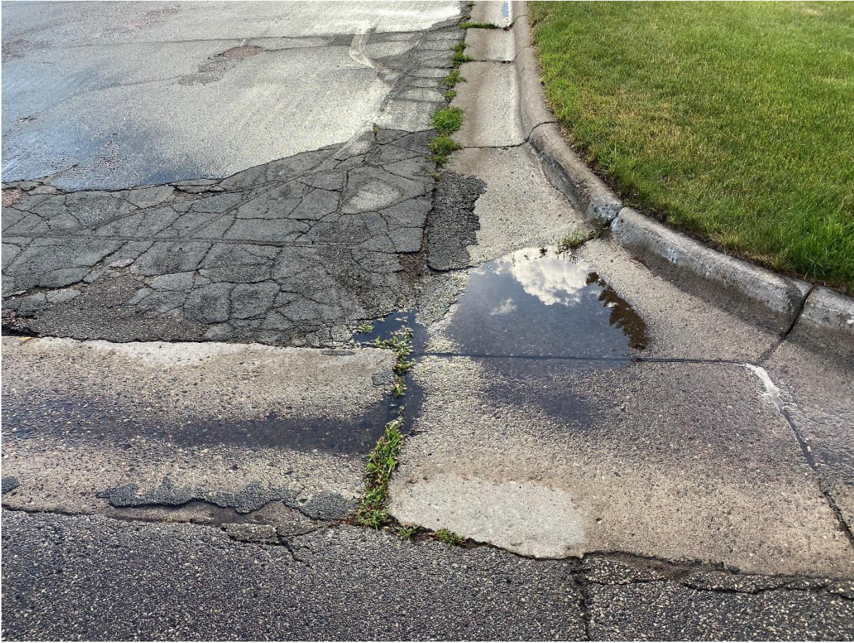
3 rd St NE at 7 th Ave NE- ponding, damaged curb.
