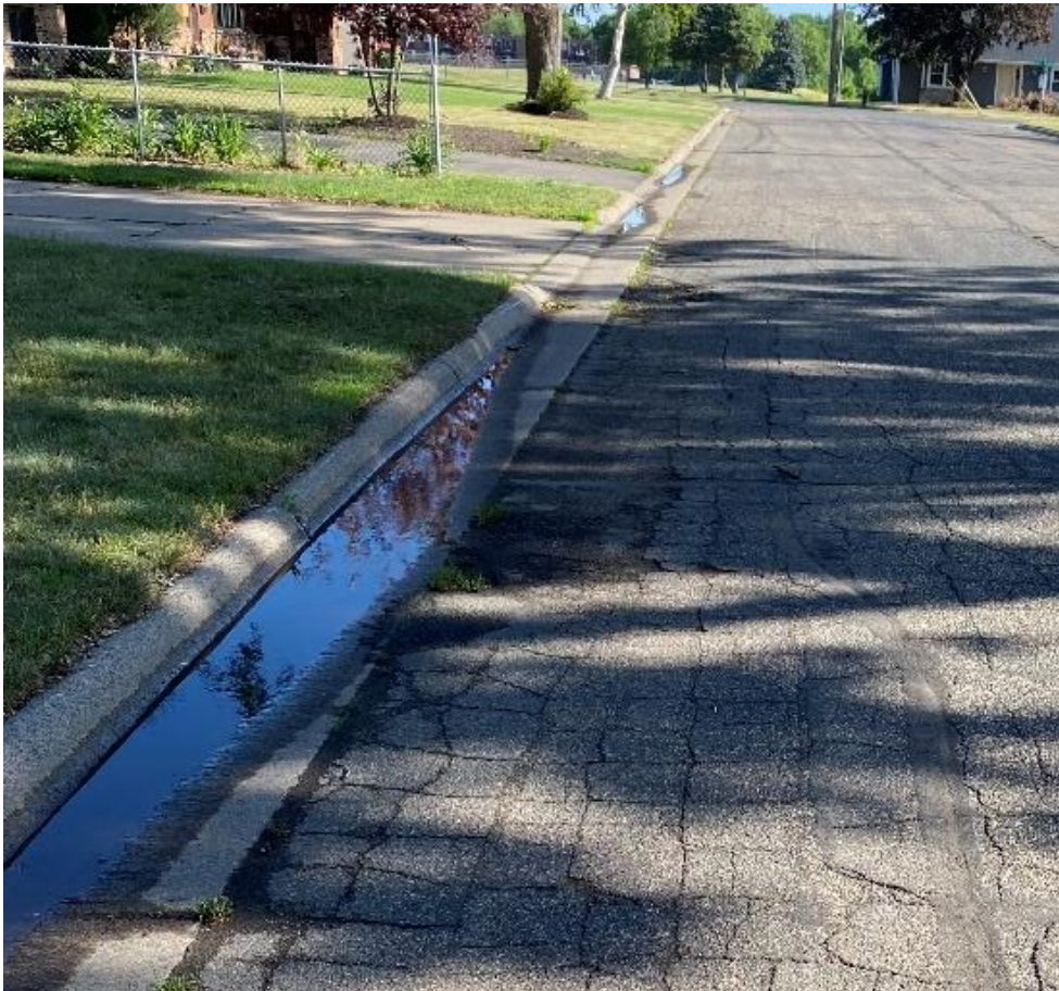
209 8 th Ave NE- ponding.
