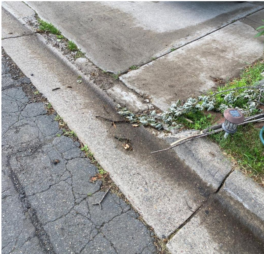
808 3 rd St NE- damage to curb.
