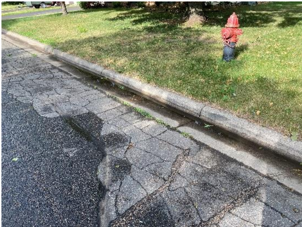
201 9 th Ave NE- ponding.
