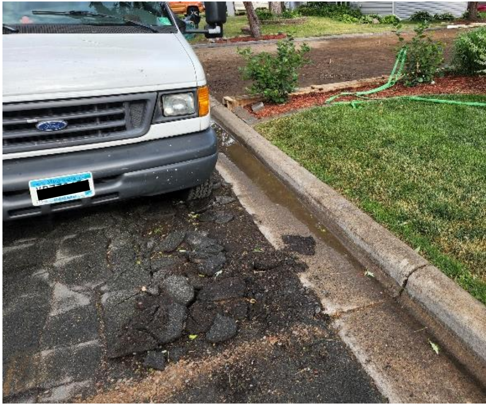
817 3 rd St NE- ponding.
