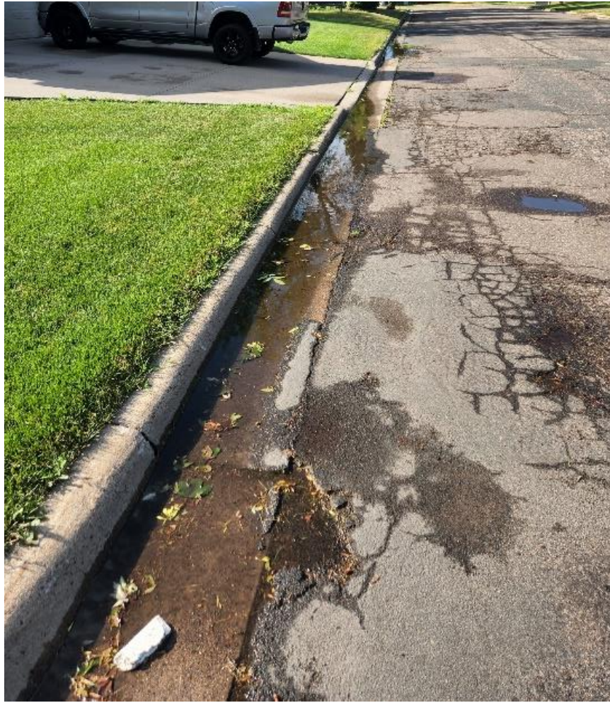
16 8 th Ave NE- ponding
