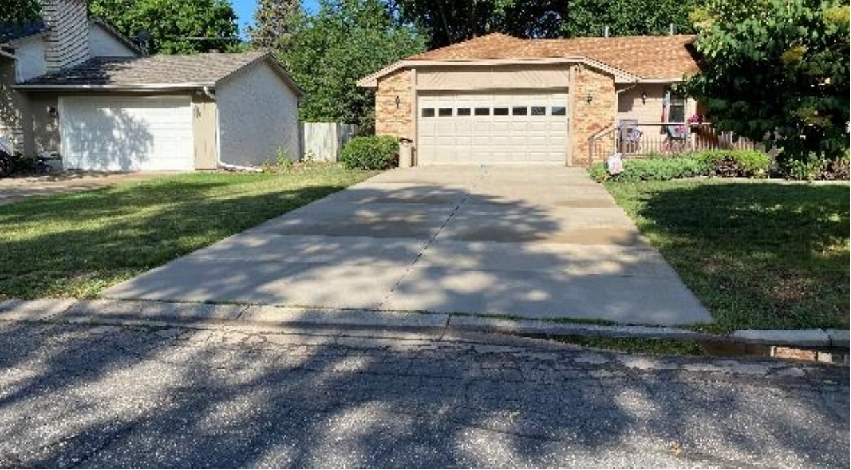
201 8 th Ave NE- ponding.
