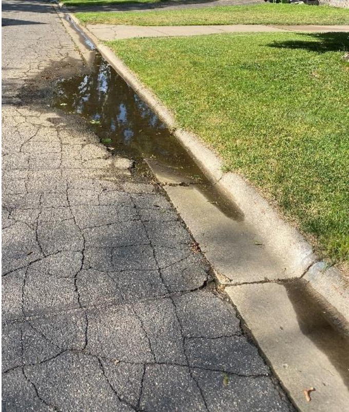
9 8 th Ave NE- ponding.
