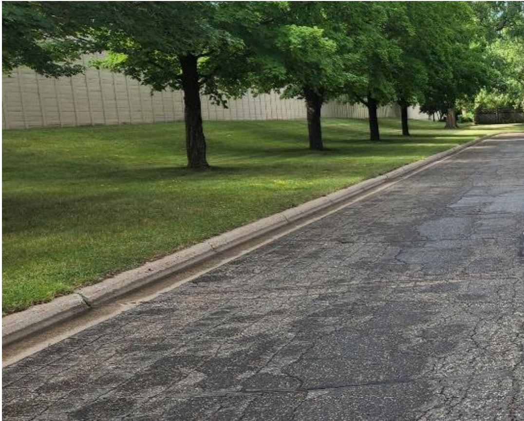
Across from 109 9 th Ave NE- ponding.
