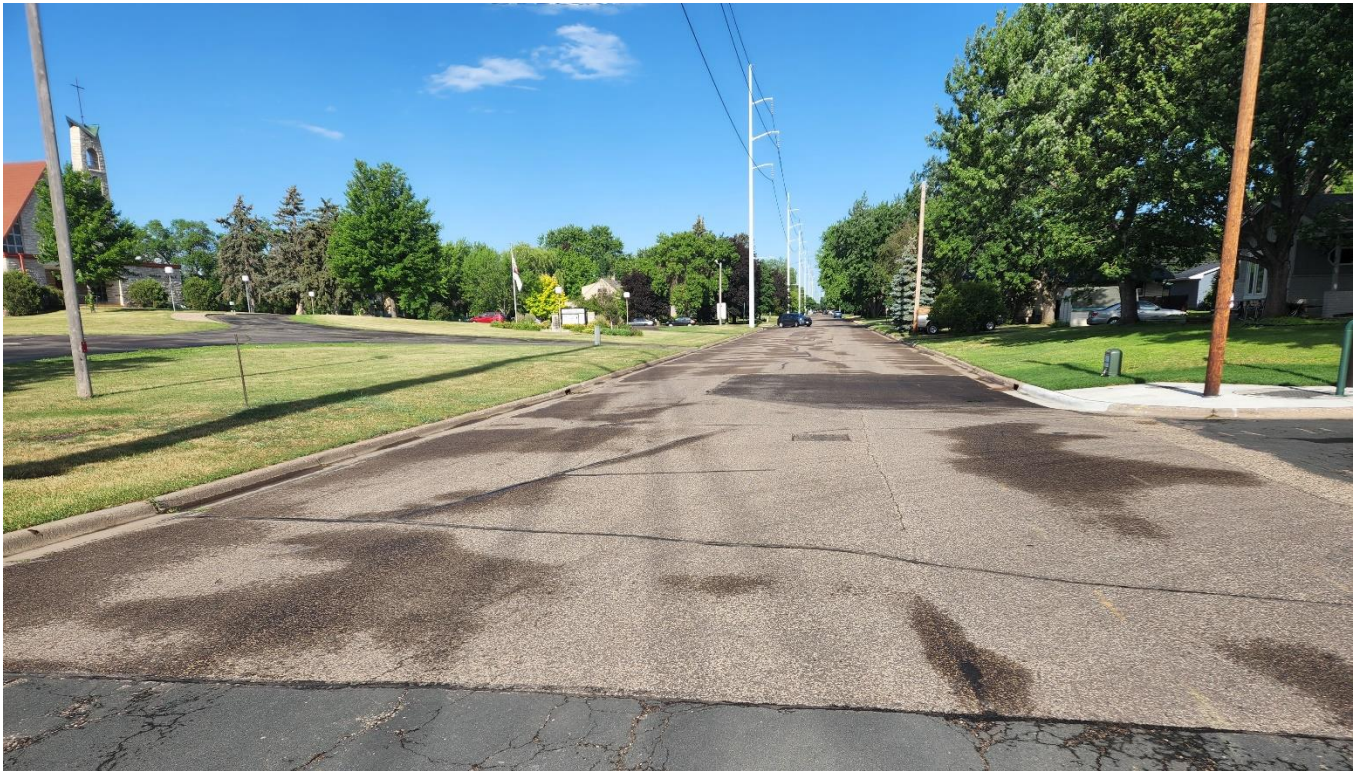
Broadway St E at 8 th Ave NE- ponding.
